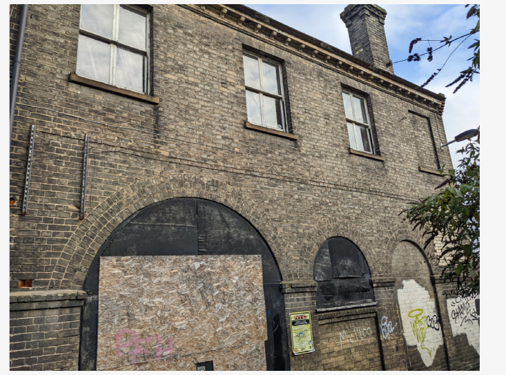
P1 - This wall of the public house is preserved but with the exterior becoming the interior.
