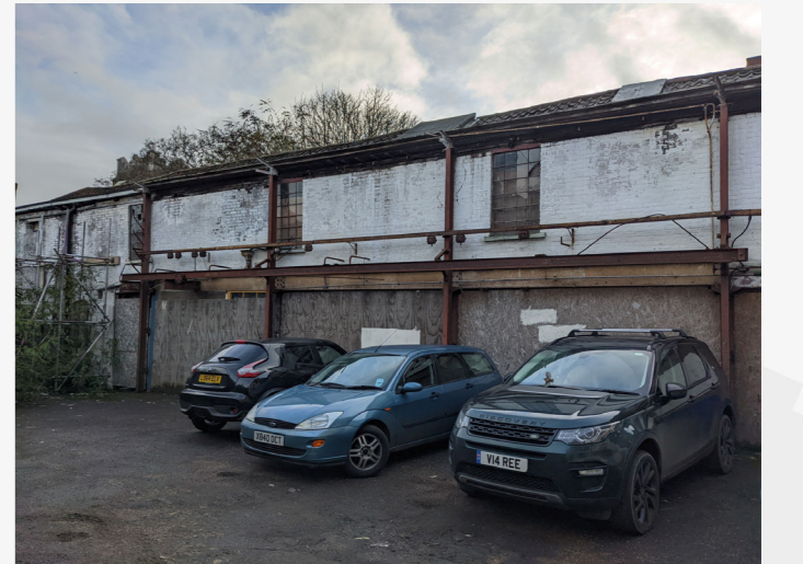
P3 - This wall is too delapidated to be preserved, but will be rebuilt as an internal wall.
