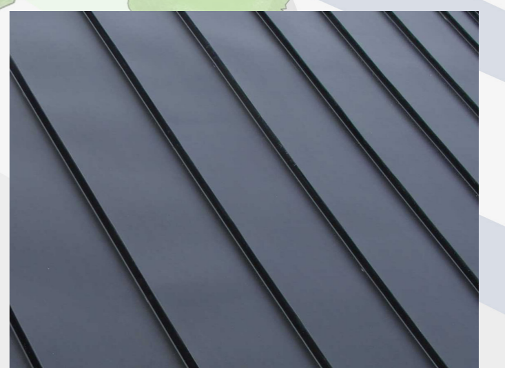
Rolled zinc roofing is used for the new additions, providing a contrast to the steelwork and resembling the traditional black tile roofs.
