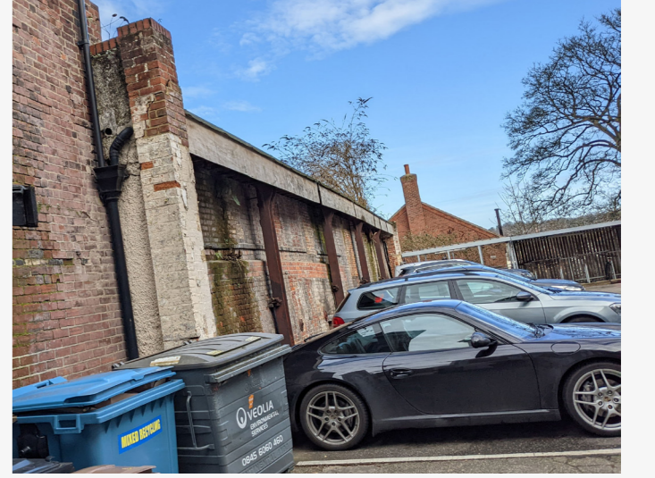
P2 - The south wall including steel columns are retained, and used to support the new roof.
